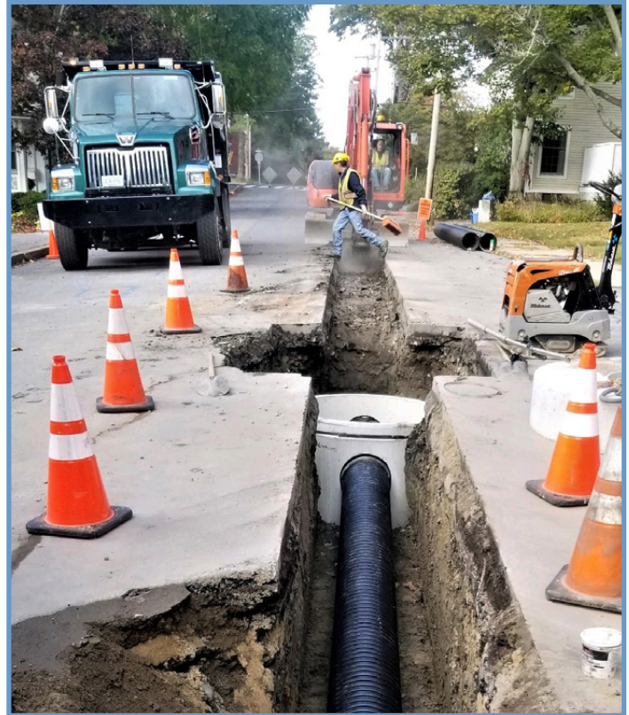
The crew works on a stormwater separation project on North Street in September of 2019
